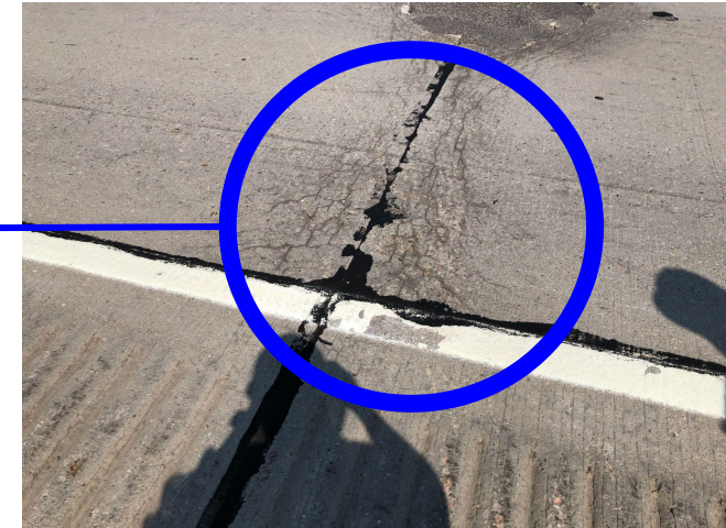
Alkali-silica reactivity (ASR) distress
